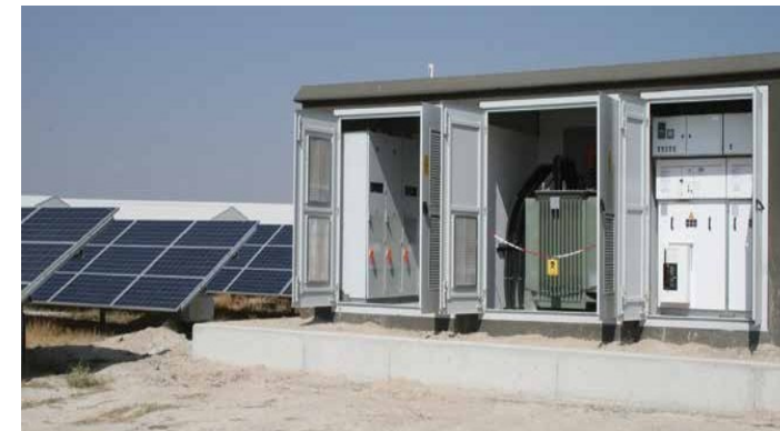
Recon Station (RST)
